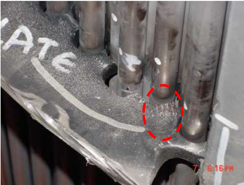
FAC appearance on worn tube support plate
