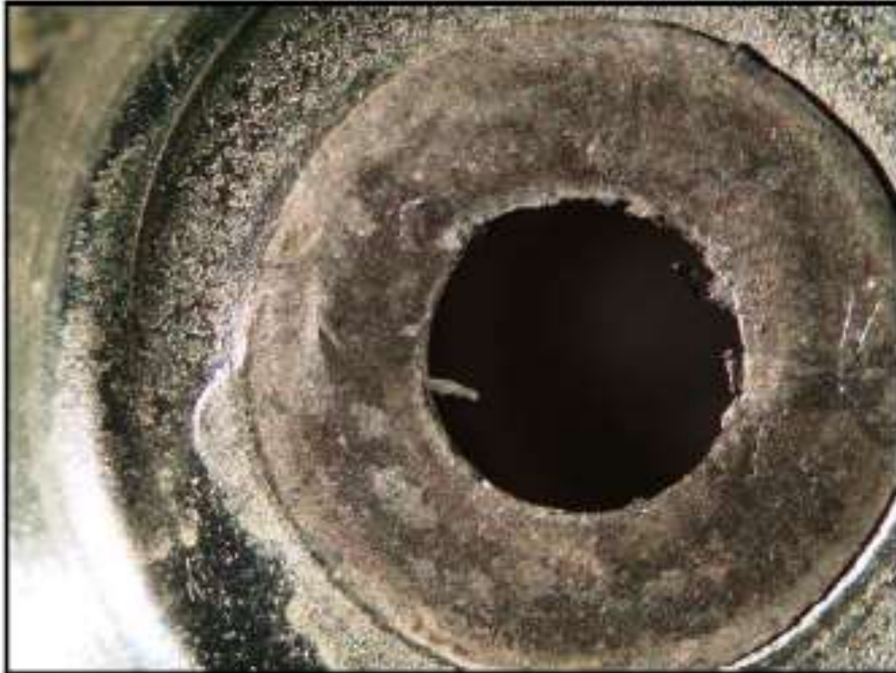
Photograph 8 Dead Space on one of the End Plates Showing Small Cast Material Flakes that Could Easily be Dislodged
