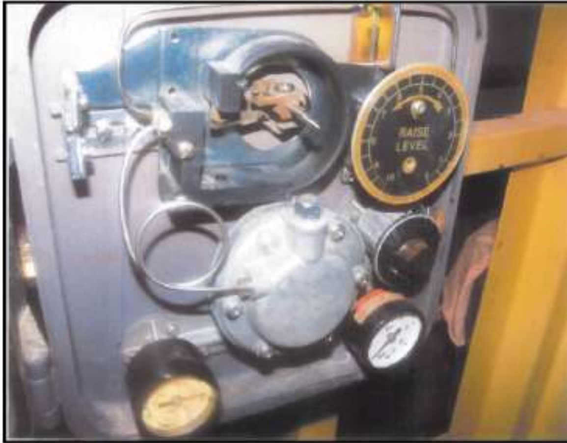
Photograph 1 Field Photograph of the Actual Controller/Transmitter Note: Level Set Adjustment Handle was Out of Place (Found Behind Dial)
